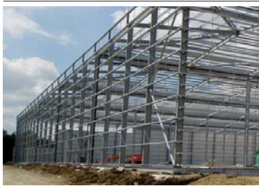
During the half year we redeveloped two Italian facilities at ProLogis Park Lodi for CEVA Logistics, adding 11,100m 2 and extended our Blois distribution centre in France by 11,000m 2 at the request of Redcats.
